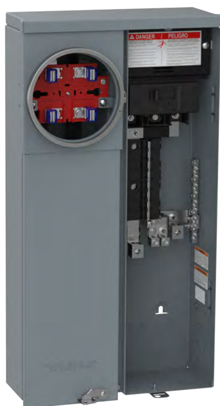
QO Meter Main
